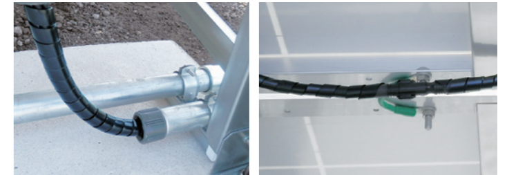
Protected from damage, just by wrapping on wires.
