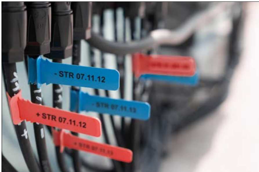
TAGPU LOOP - Cable marking solutions for labeling on the inverter.
