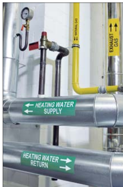
Large and highly visible pipe marking.
