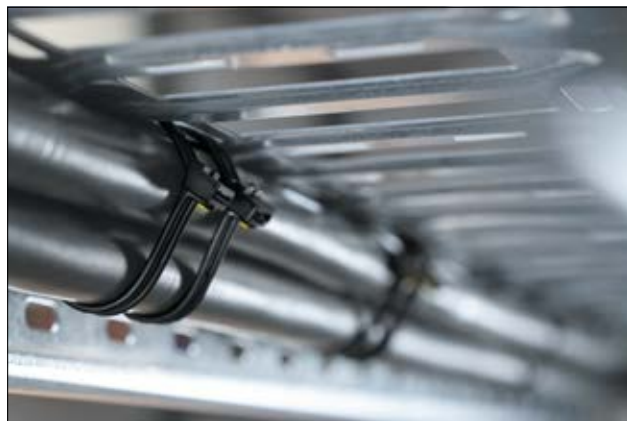
KR-Series ties applied on a cable tray.
