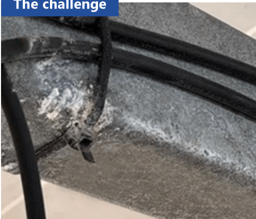
Typical zinc chloride corrosion 3 years after installation at a location near the Pacific Ocean
