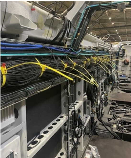
Dense cable bundles during temporary installation phase
