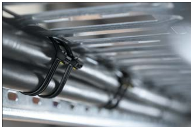
KR-Series ties applied on a cable tray.
